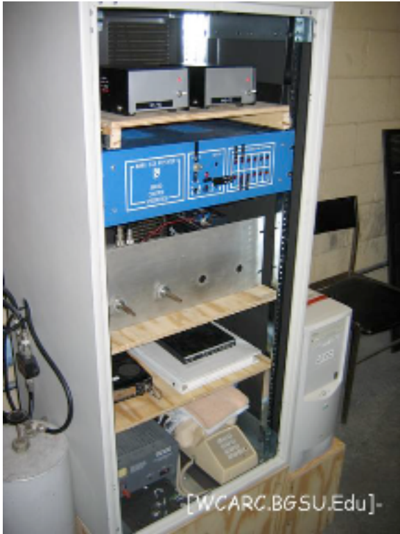
Receive Site Cabinet
