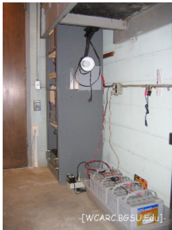
Transmitter Rack with Emer- gency Back-up Batteries
